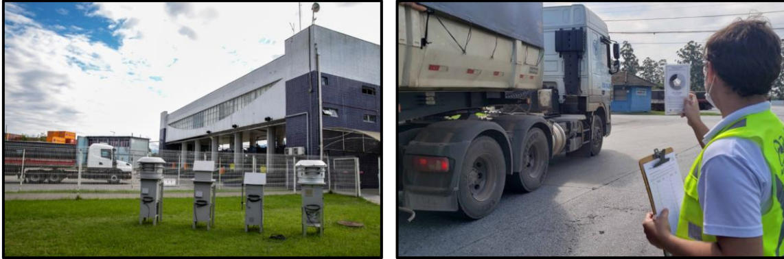
Figure 17. Equipment installed to monitor air quality in the port surrounding and black smoke monitoring with the methodology known as “Ringelmann scale”.
